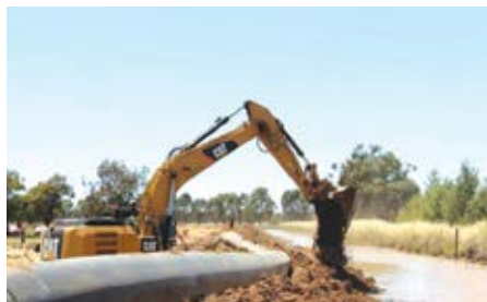
Equipment working on a section of the project area near Numurkah in Victoria. This included decommissioning 1,100 m of channel, one regulator, a road crossing and 13 outlets as well as four meter upgrades and the installation of 100 m of pipeline.
