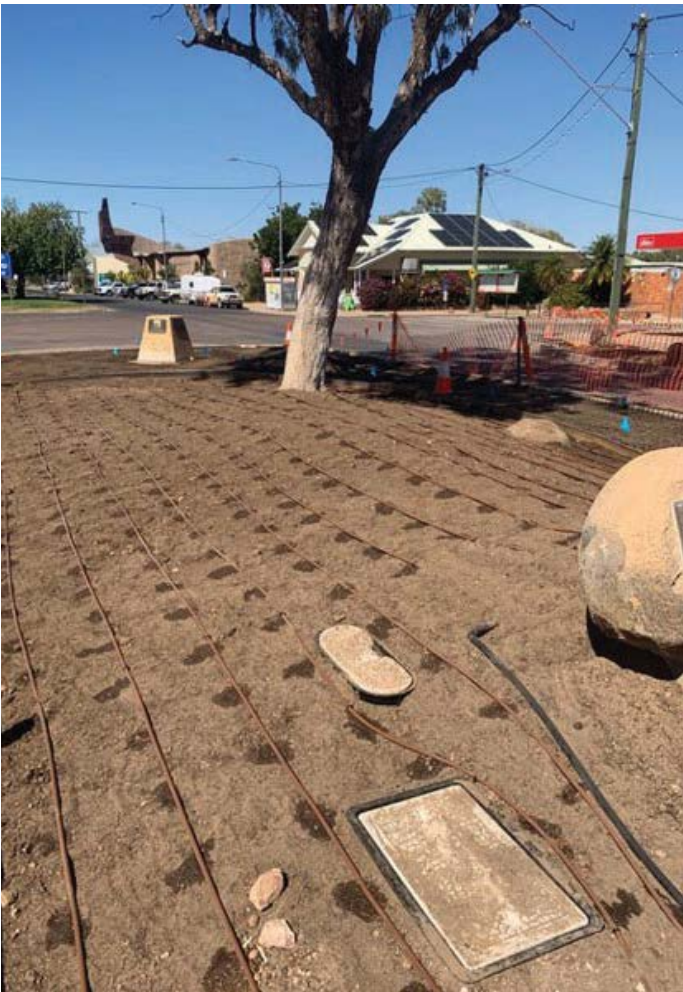
Drip line installed as part of the upgrade to the main street of Winton.
